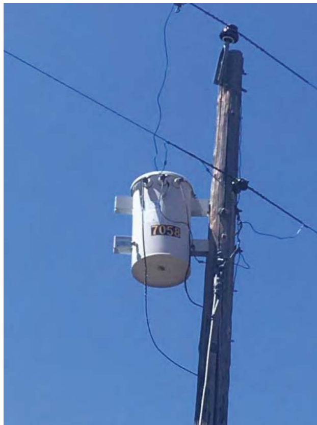
Description: Transformer labeled "no PCB"
