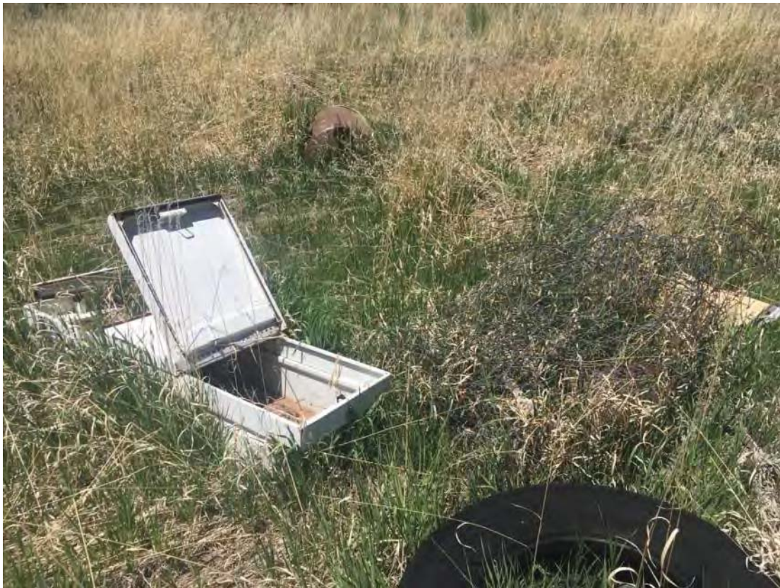
Description: Drainage debris
